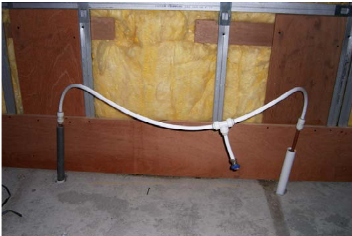
Figure 14 Ply backing on lightweight frame, to hang services and minimise penetrations through insulation and air tightness barrier
